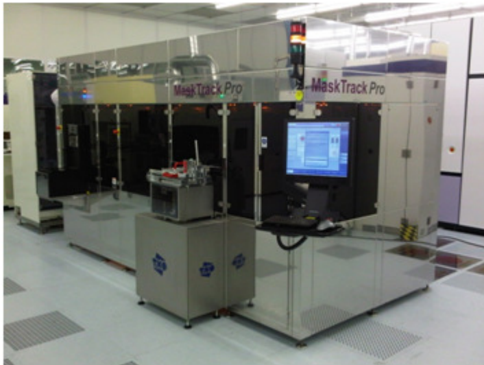
MaskTrackPro installed at imec
